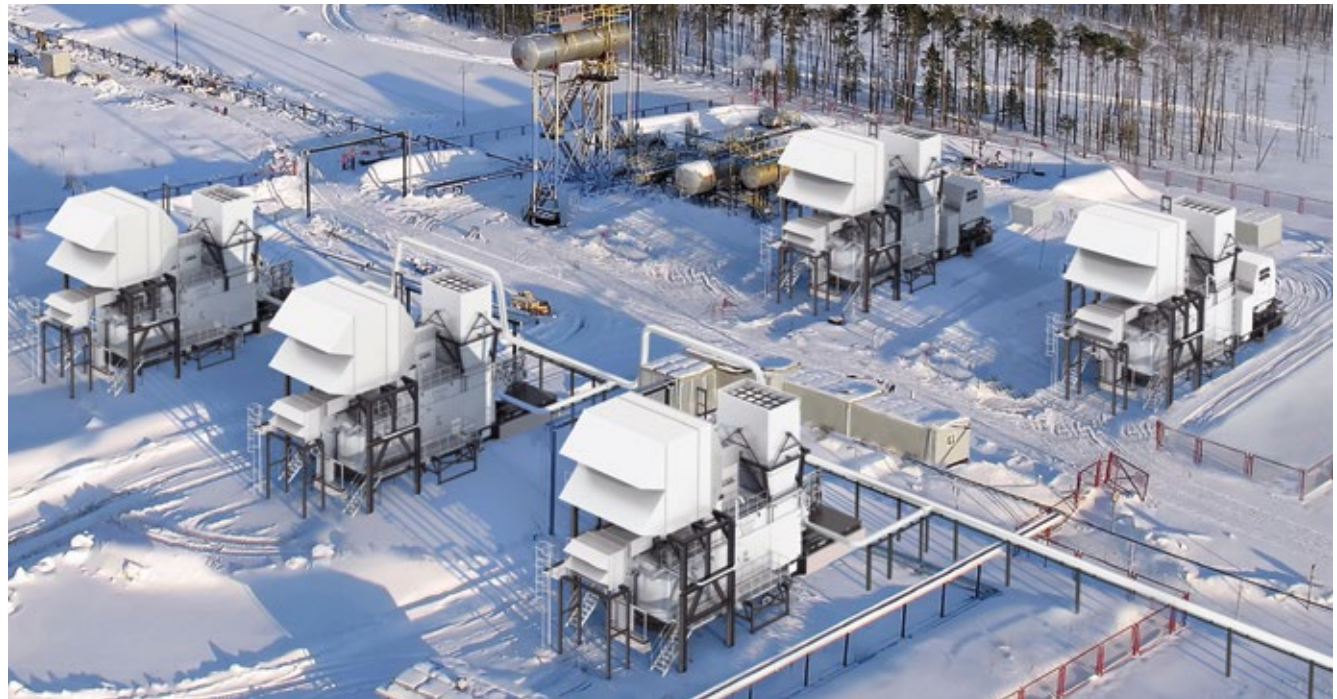
SGT-600 installation for both mechanical drive and power generation
